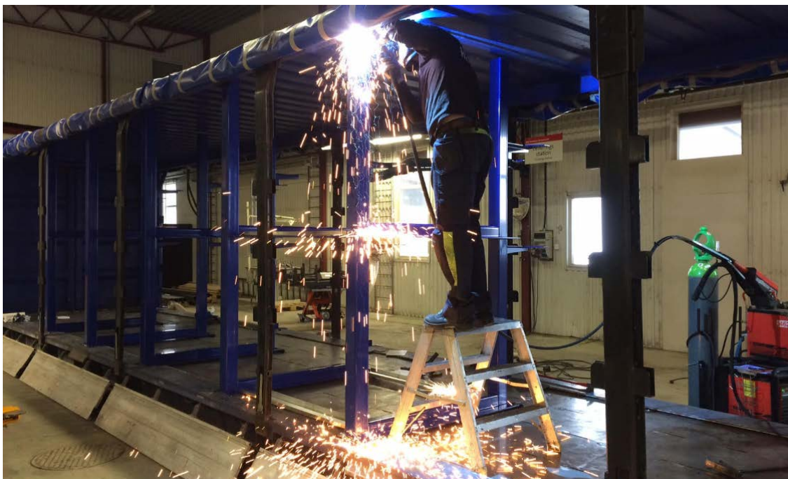
Welding of a motor stand into a container for the PWR BLOK, March 2018
