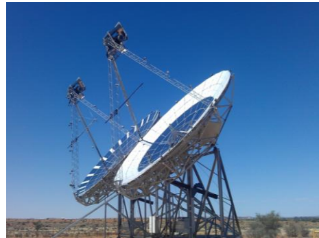
Ripasso Energy Stirling Dish modules during commissioning, evaluating different mirror area
