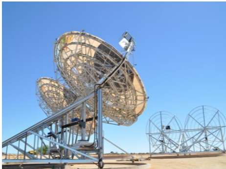
Ripasso Energy Stirling Dish modules under installation in Upington, RSA (2 x 30 kW per module)
