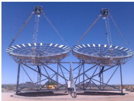
Ripasso Energy Stirling Dish modules in operation at Upington, demonstrating the new world record
